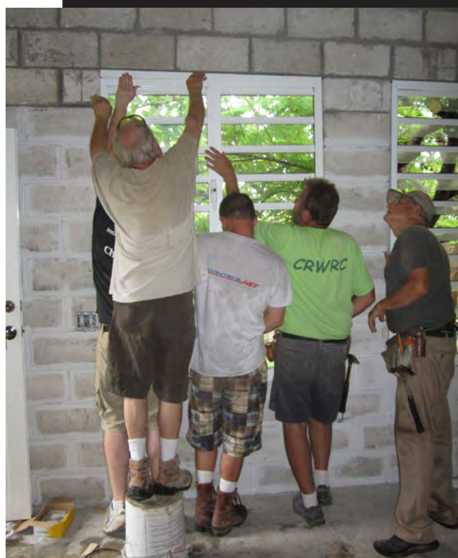
Volunteers putting up an addition to missionary Ben Hopp's house in Haiti
