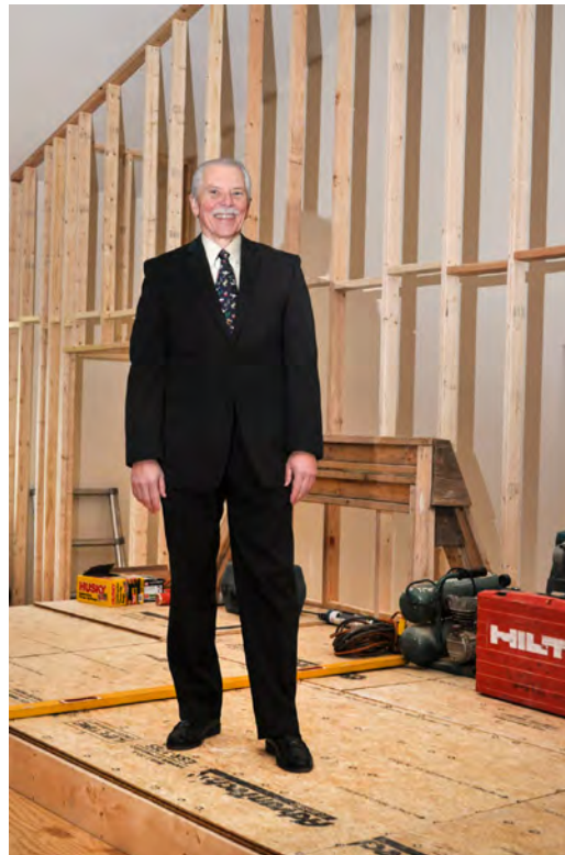
Elder Glenn Taylor, the primary contact between Bethel Presbyterian Church and the contractors, standing close to where the pulpit will be placed
